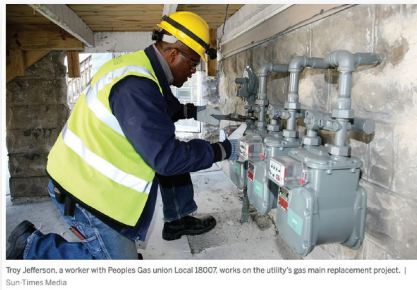
Troy Jefferson, a worker with Peoples Gas union Local 18007, works on the utility's gas main replacement project. | Sun-Times Media
